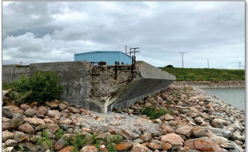
Figure 1: Deterioration of the pump station's substructure
